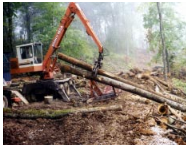
Figure 4: Poor location of the loader resulting in operational delays when loading out the truck.
